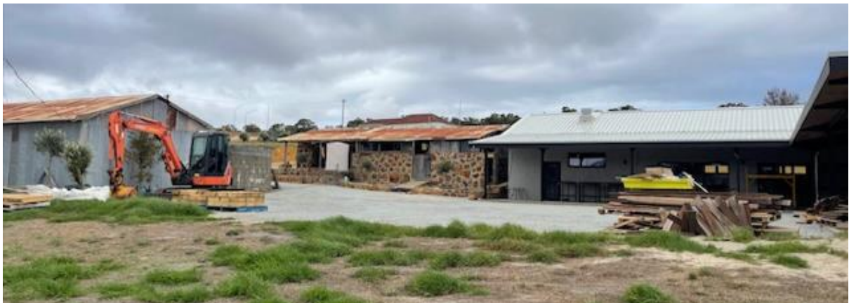
Work in Progress showing Shed, Old Ironstone Dairy & New Building with Courtyard in Centre
